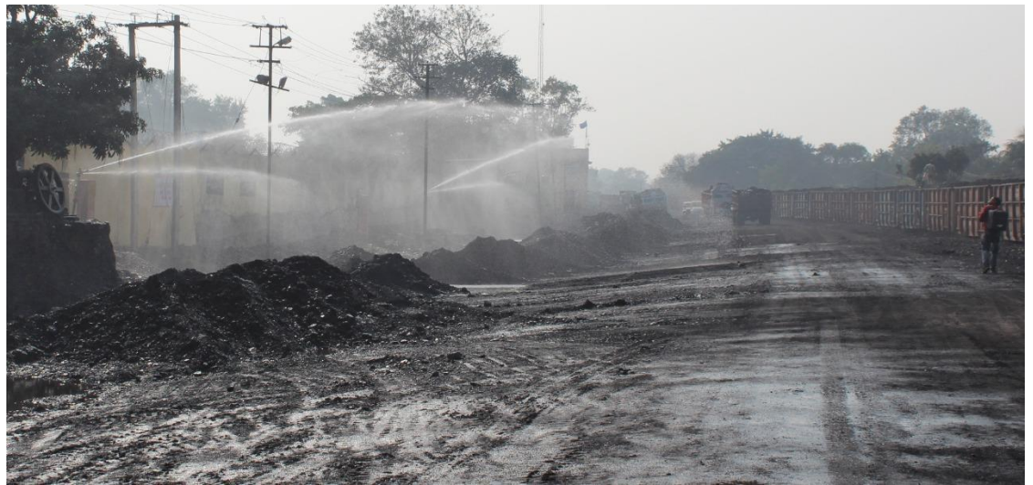
Fixed Type Water Sprinklers at JK Nagar Railway Siding
